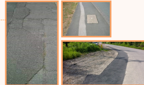
Evidence of service trenches/ scarring
