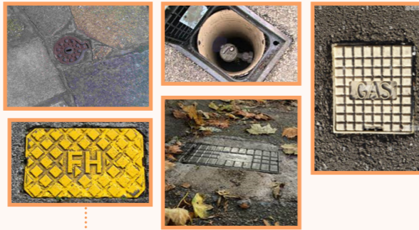
Stopcocks/fire hydrants/meter covers/toby box
